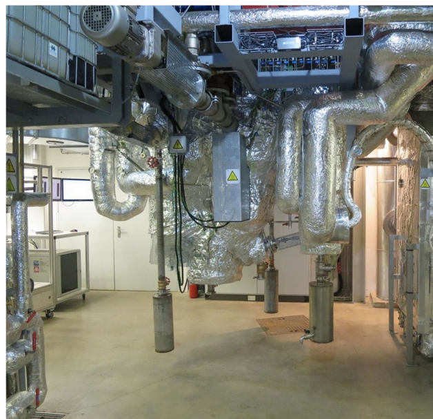
Fig. 7 Picture of the pilot plant with thermal insulation and ash containers (lower floor)
