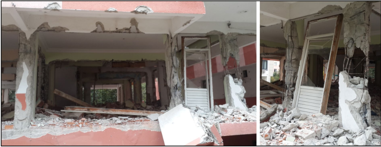
Fig. 9 Two heavily damaged corner columns for HD-I
