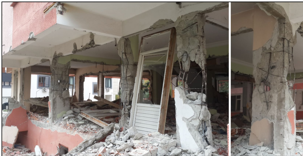
Fig. 11 Heavily damaged three columns for HD-II
