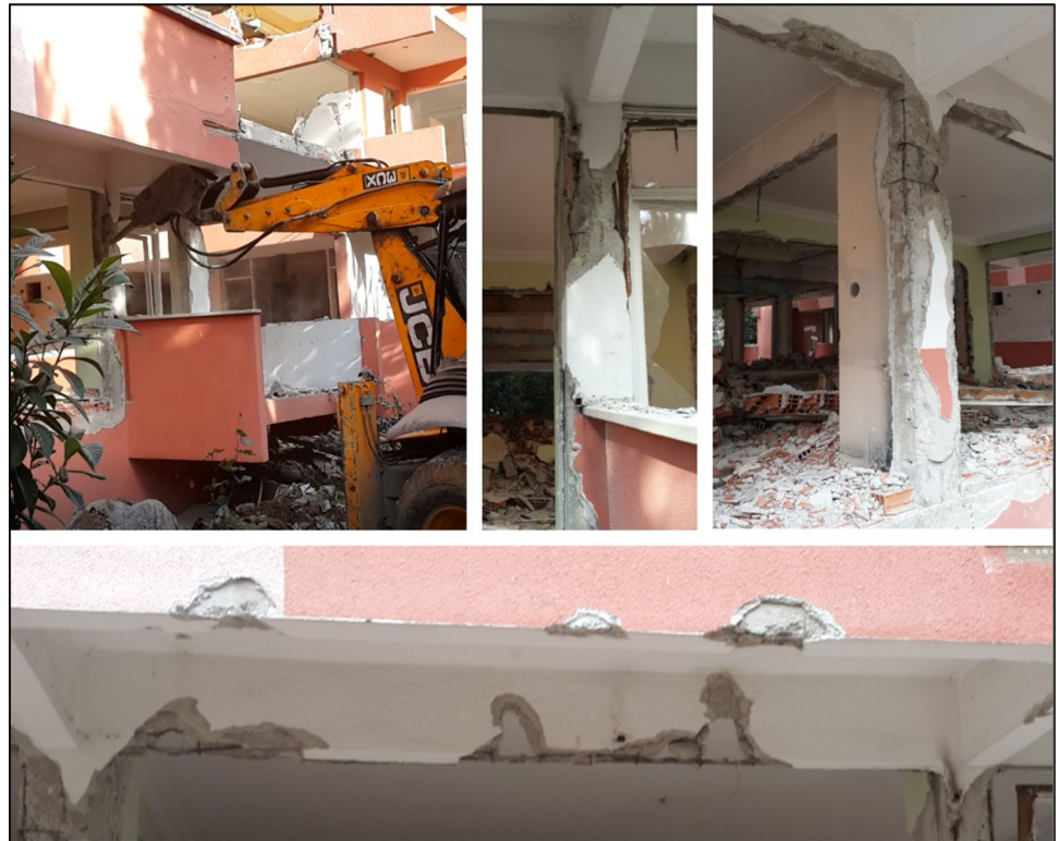
Fig. 7 Three damaged columns and one beam for moderate damage (MD)
