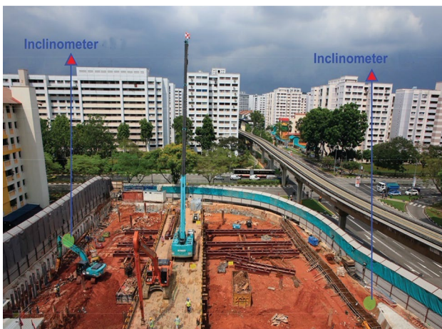
Fig. 6 Bukit Panjang hawker center excavation. Courtesy of Lian Soon Construction PTE LTD
