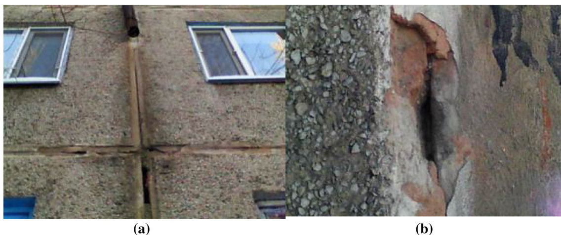
Fig. 12 Examples of metal joints corrosion in PC damaged buildings. a/b – signs of concrete colour change due to corrosion
