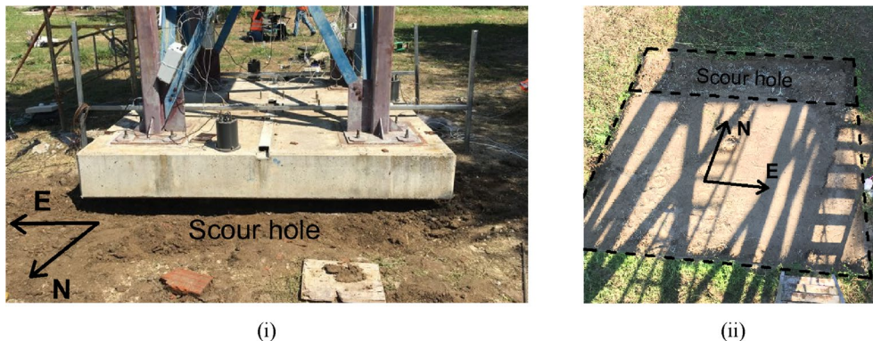
Fig. 5 i Excavation of the soil under the foundation, ii scour hole shape at the end of the final test
