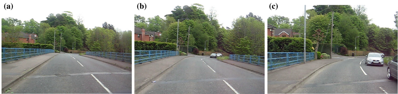
Fig. 10 Bridge expansion joints at crossing over M1 motorway on Dunmurry Lane on test route 2; a west entrance, b centre, c east entrance
