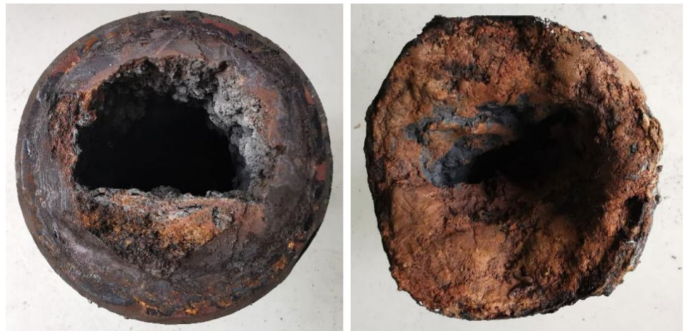
Fig. 1 Morphologies of deposit at front end and rear end of breathing pipe
