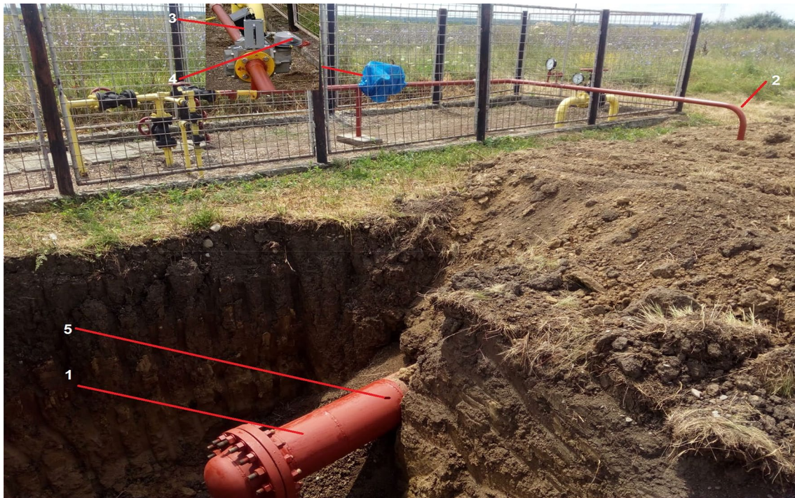
Fig. 3 Natural gas leaks calculation experimental stand: 1—buried pipeline; 2—filling nozzle; 3—rotary piston counter; 4—absolute pressure transducer; 5—defect
