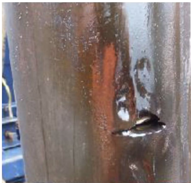
Fig. 7 Metal Piping Crack due to Solids (Pastre and Fastovets, 2017)
