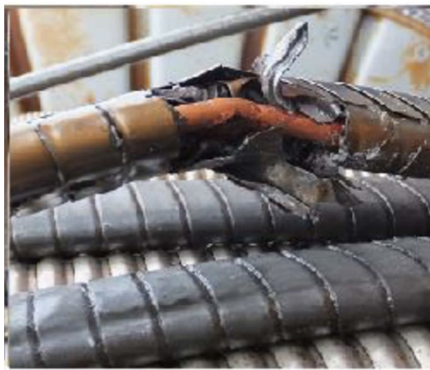
Fig. 5 Example of ESP Assembly Cable Failure (Pastre and Fastovets, 2017)
