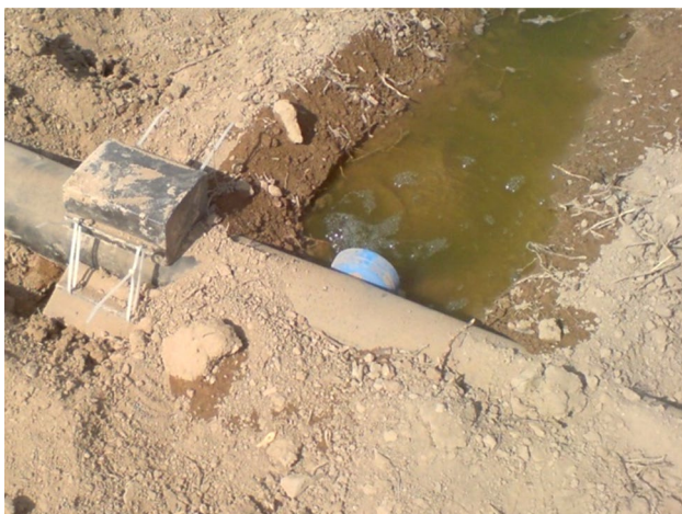
Fig. 1 The magnetic machine mounted on the valve pipe
