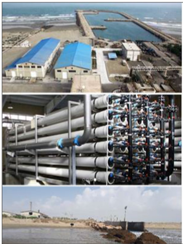
Fig. 2 Konarak RO desalination plant
