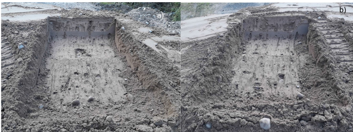
Fig. 5 Trench a was dug by a human driver, and trench b was dug by a semiautonomous excavator
