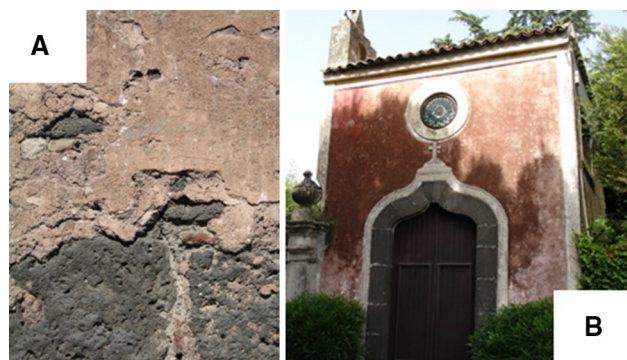
Fig. 3 a Detachment of mortar based on ghiara; b Original plaster application in San Salvatore church in Viagrande, Catania, Italy
