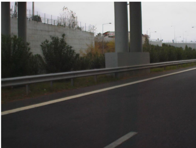
Fig. 3 Bridge column in contact with guard rail
