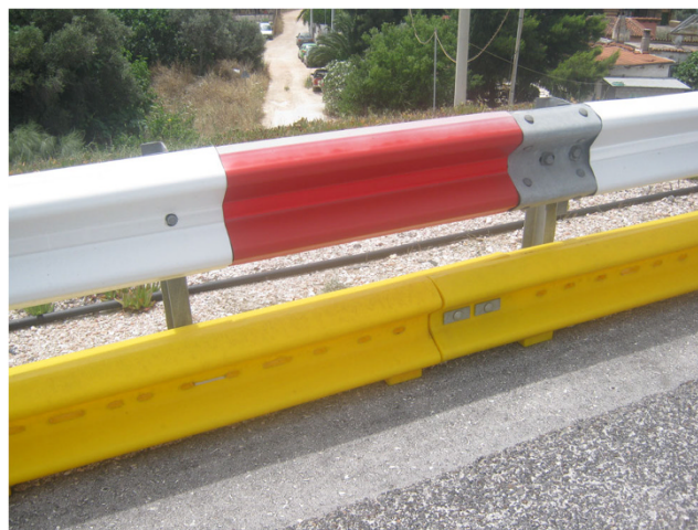
Fig. 5 Secondary rail to protect motorcyclists
