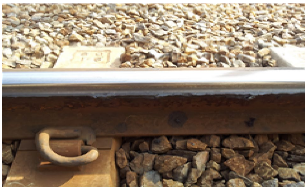
Fig. 9 Head check of high rail gauge in curve
