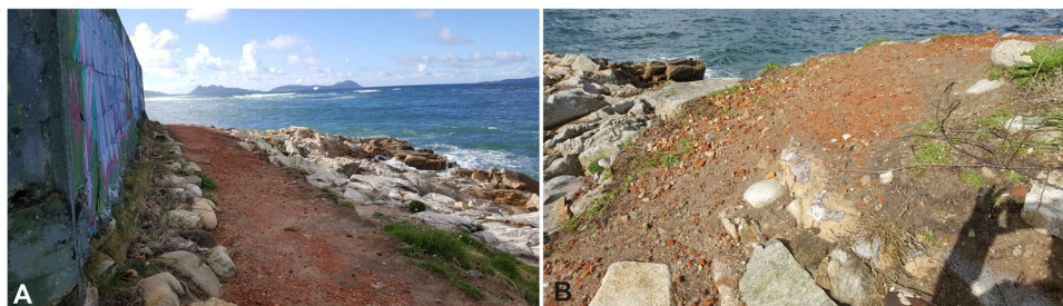
Fig. 24 A View from the east of the intervention area, taken in March of 2018. B Detail of the mortar area, where the loose of material can be seen
