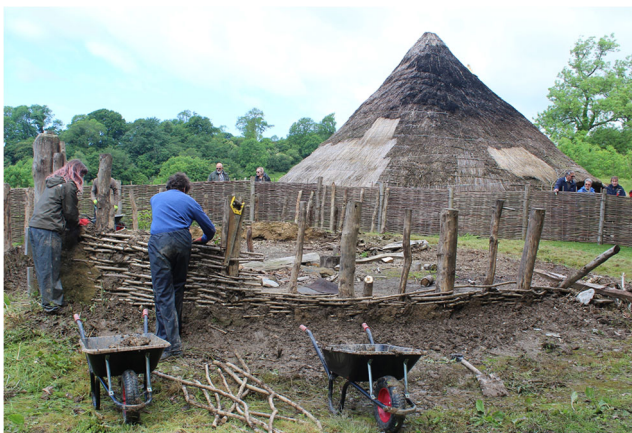
Fig. 13 Partially standing Cookhouse wall with wattle and daub and slumped wall materials
