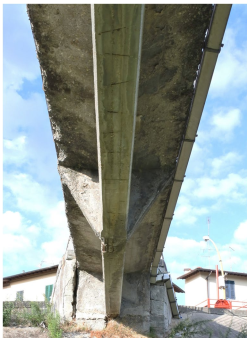
Fig. 7 Walkway, diffuse concrete corrosion
