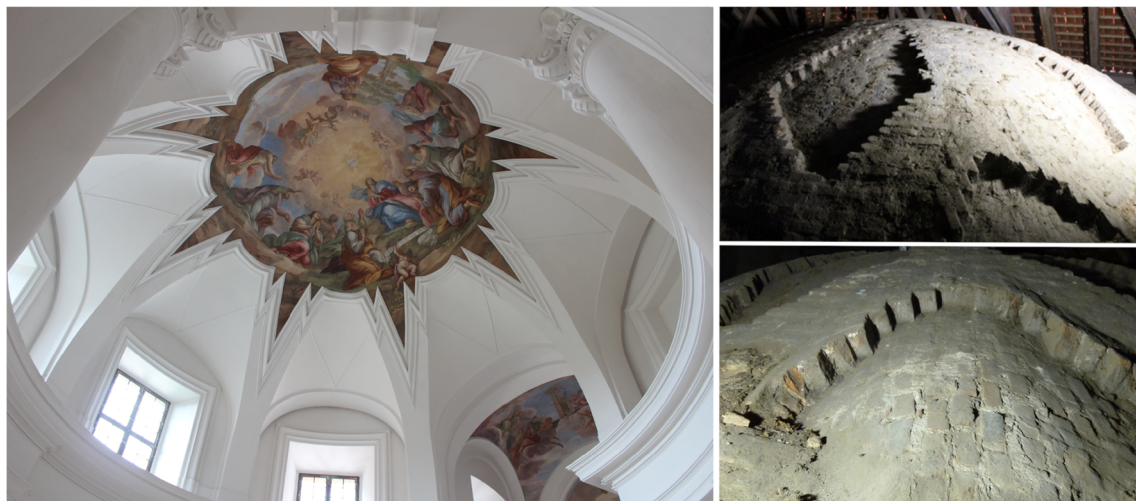
Fig. 2 St. Bernard's chapel. Left: Vault intrados: eight lunettes and ribs, central frescos by artist J. A. Pink. Top right: vault extrados: Y-shaped ribs with interlocking bricks on the two edge of the lunettes. Bottom right: lunettes brick arrangement
