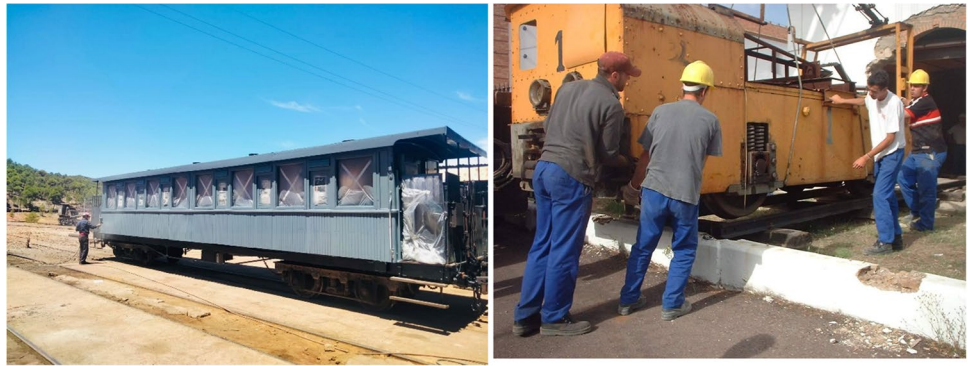
Fig. 6 Left, construction of a covered car on an F1-type platform. Right, moving an electric locomotive into the museum
