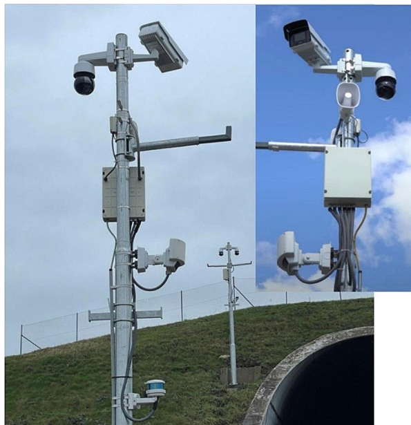
Fig. 9 Security technology for the Břežno tunnel portal mounted on a column - lidar, radar, IP horn speaker, PTZ camera tracking the detected object, static camera monitoring the portal - in order from the bottom (Smažinka and Hrinko 2022)
