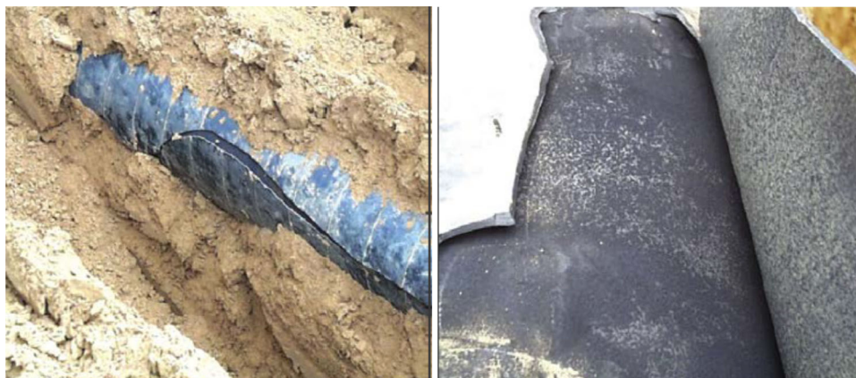
Fig. 6: Common field failures of 3LPE coating systems 16
