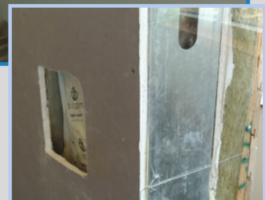
(Inset): A cross section of the atrium’s walls showing the installation of a phase change biomaterial over the insulation for thermal massing.
