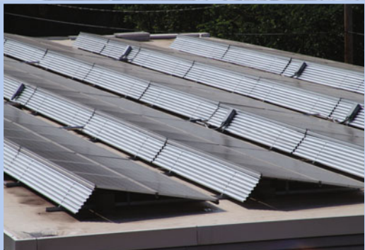
(Second and third photo): To operate efficiently in such a limited space, the CSL’s solar installation was split into three major arrays, covering two separate buildings and a ground array on the edge of a hillside.
