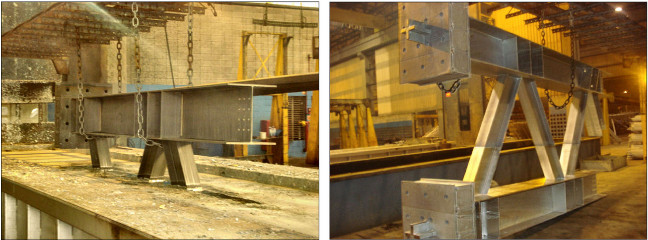
Fig. 1 Double immersion procedure used for the hot galvanizing of the 226 trusses for the assembly of the pipe rack
