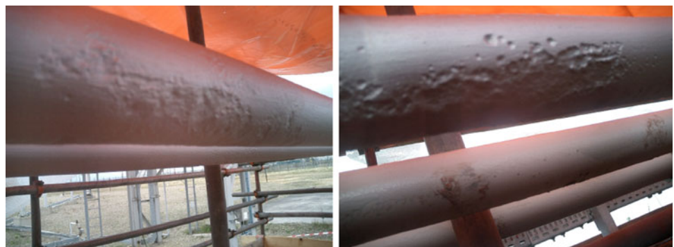
Fig. 2 CUI degradation on hot oil lines showing multiple coalesced pittings from 2 to 10 o'clock positions
