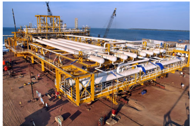
Fig. 10 Finger-type slug catcher—large surface area available for solid deposition, less inspectability and maintainability
