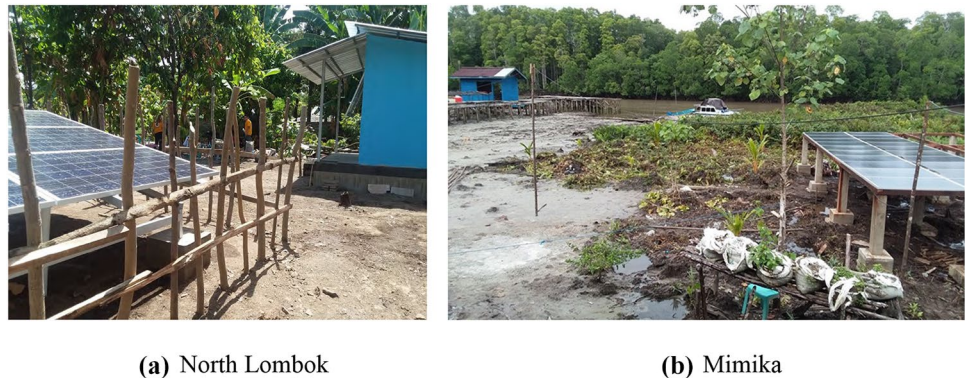
Fig. 3 The implemented solar photovoltaic (PV) system facility for ice making for fishermen (Source: author's collection)
