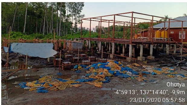
Fig. 7 A community store under construction in Mimika, Papua that builds on the availability of solar energy (source: Maria Bintang Laut, NGO)
