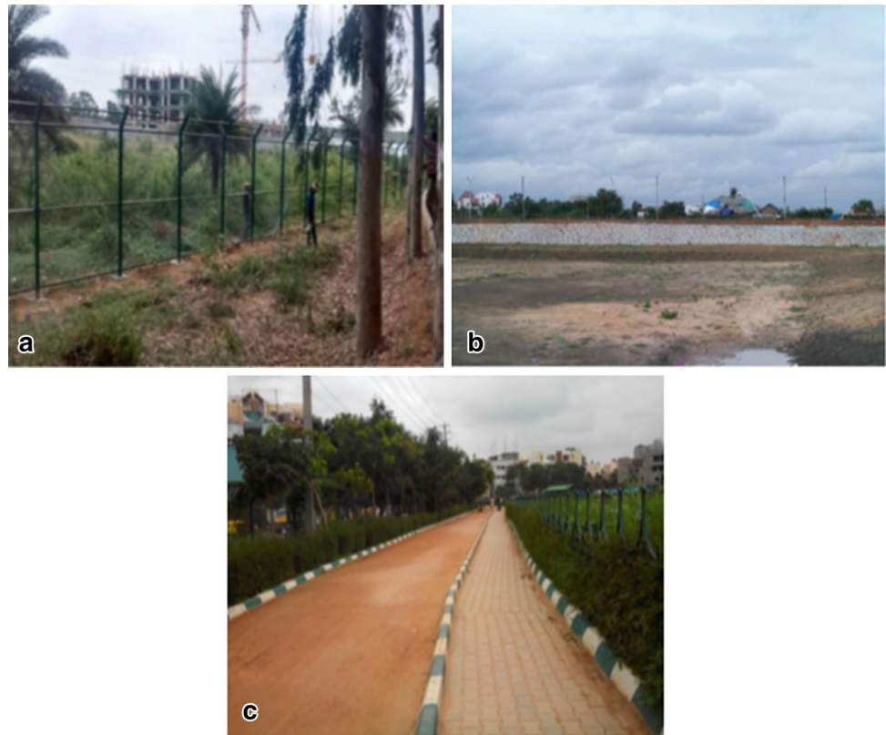
Fig. 1 Initial stages of lake restoration. a Fencing. b De-silting and bund formation. c Paving bund as walkway
