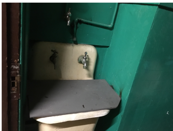
Fig. 2 Covered broken sink at SRO #8
