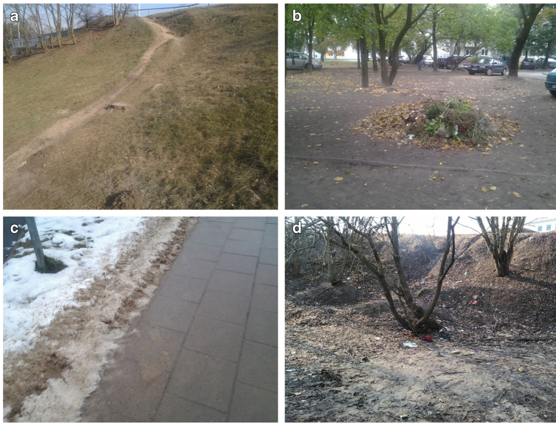
Fig. 1 Soil degradation and sediment accumulation in roads in Vilnius (Lithuania) a road trail, b municipal clean-up activities, c sediment accumulation, and d rill and gully formation
