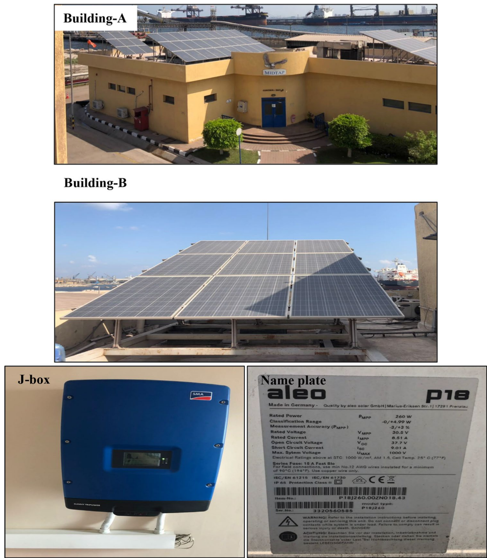
Fig. 5 Solar panel installation on building A and building B. On the bottom, the junction and name plate of the installed panel
