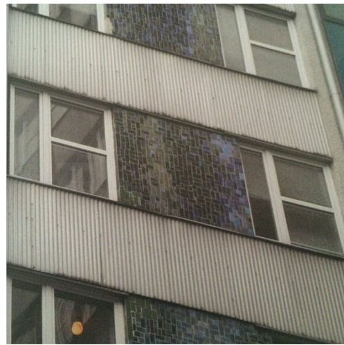
Fig. 1 Facades of the Faculty of Building Services, Hydro and Environmental Engineering (KODnZEB, 2015–2017)
