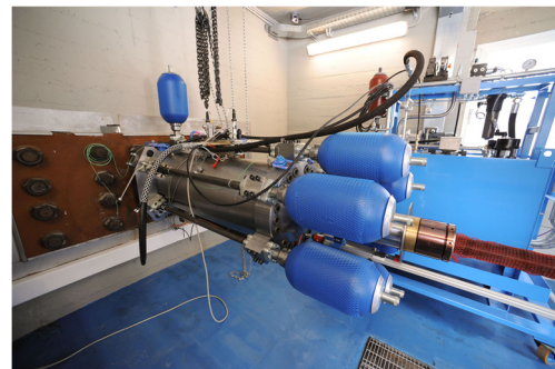
Fig. 9 West cylinder and hydraulic pumping station
