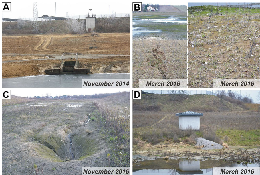
Fig. 5 Examples of operating problems in the RHTS–variant 2 (2014–2020): A ) the risk of influx of the products of erosion from the steep northern slope; B ) rill and surface erosion on the escarpments of the reservoirs; C ) piping in the bottom of the western infiltration reservoir; D ) too high elevation of the intake of water after treatment
