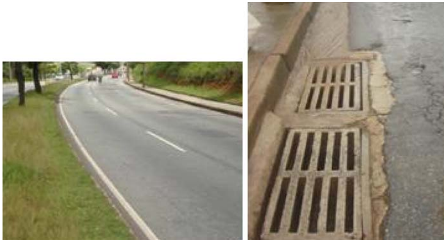
Fig. 1 Partial view of the contributing area ( left ); Inlet installed at the gutter ( right )
