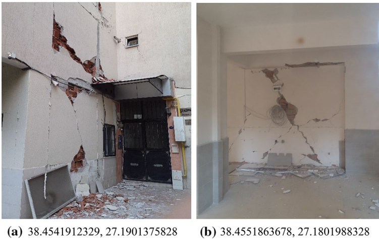
Fig. 34 Shear cracks on walls without openings
