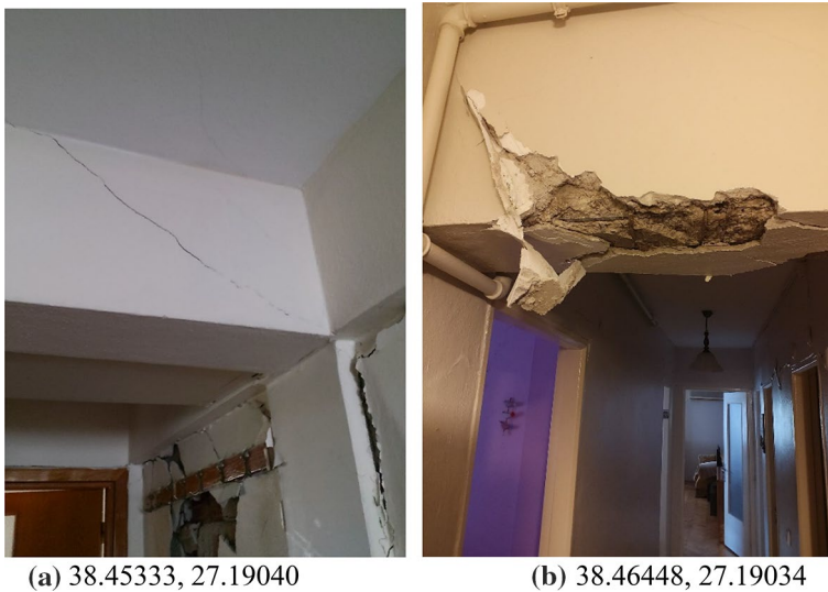
Fig. 25 Damaged beams during the September 30, 2020, Aegean earthquake
