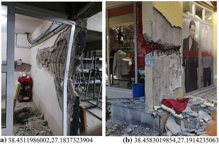
Fig. 39 Reinforced concrete shear wall damages
