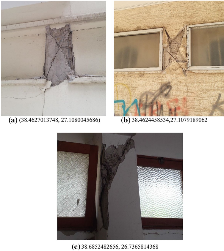
Fig. 27 Short column damages
