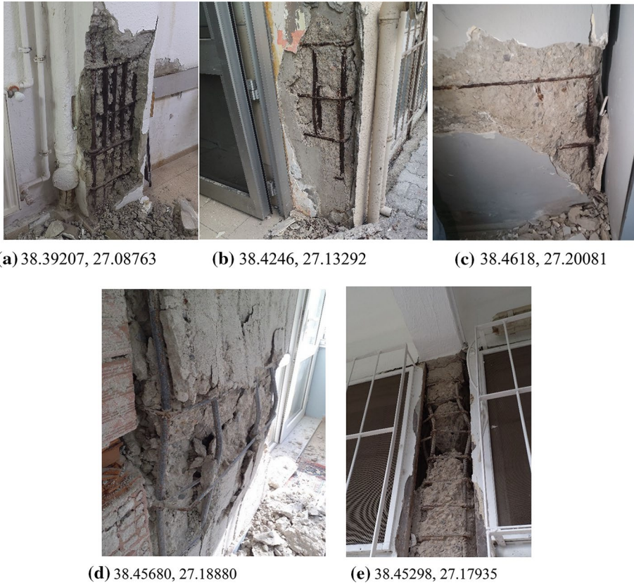
Fig. 31 Failure of column due to poor concrete quality during the September 30, 2020, Aegean Sea earthquake
