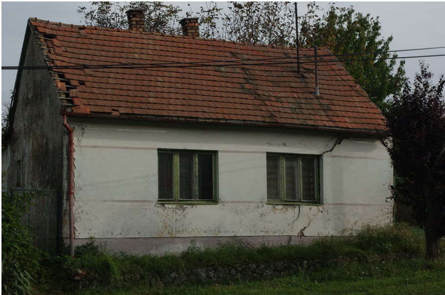
Fig. 10 Abandoned house on the active landslide mass at Dunaszekcső in October 2016 (location in Fig. 7)
