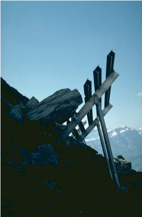
Figure 1. Snow bridge in permafrost terrain damaged by rock fall (Emshorn, Valais, 1996).
