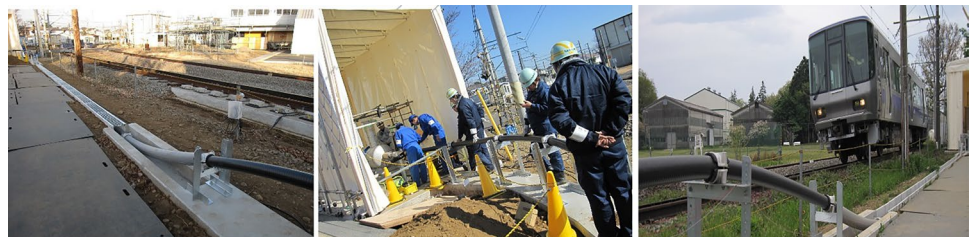
Fig. 3 31 m Bi-2223 superconducting cable installation for train run test at RTRI, Tokyo
