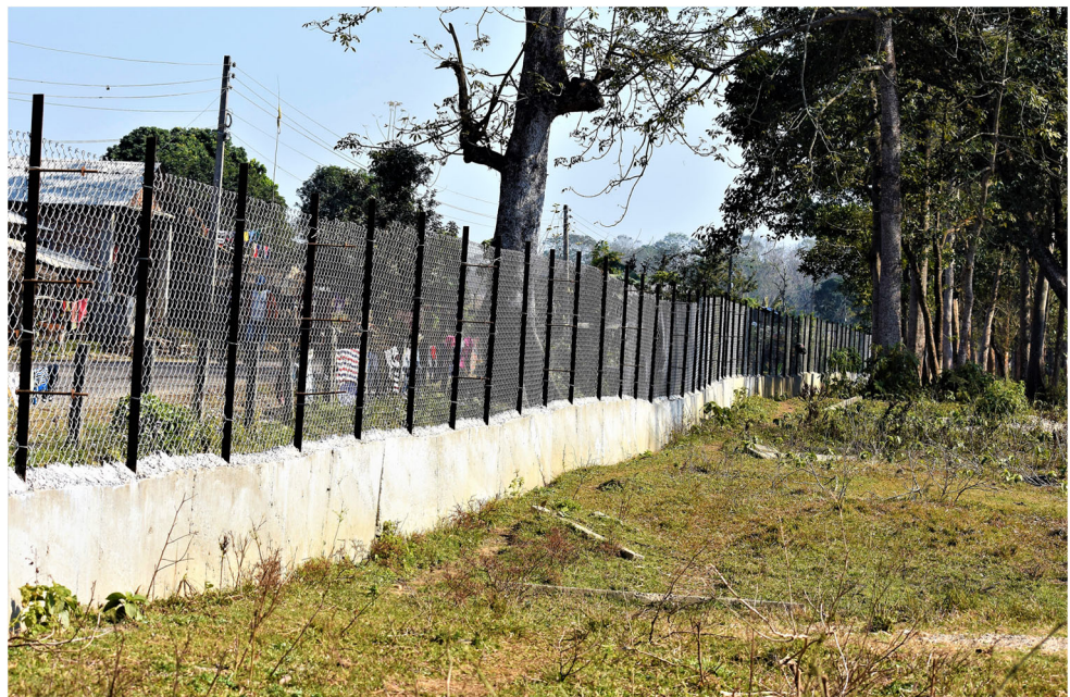
Fig. 7 An example of the mesh wire fence communities prefer to construct along the forest-settlement border. The fence has a concrete base of about 2 ft and 5 ft tall mesh wire anchored to the iron poles set in a concrete base
