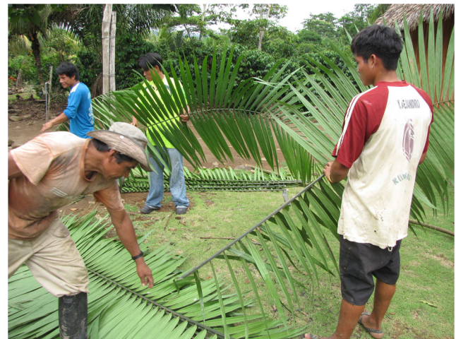
Fig. 9 Preparation of chorinashi - Oenocarpus mapora leaves for repair of the radio station roof
