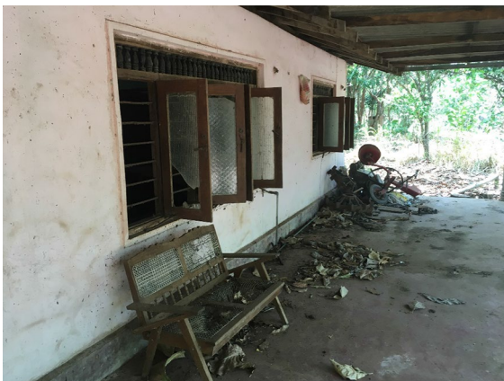
Fig. 3 Abandoned house, reportedly left by inhabitants due to HEC. Photographer: Authors
