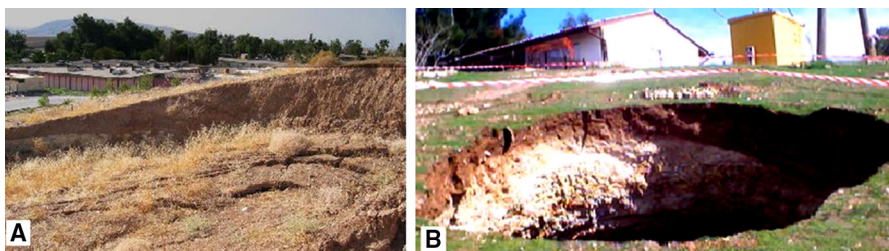
Fig. 9 The left bank sinkhole a early stage b full development stage
