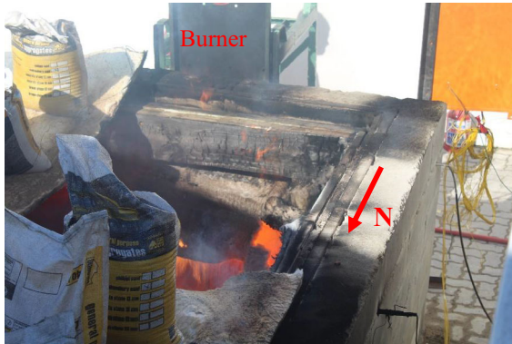
Figure. 11. Failure at the South-West corner of the SD during the preliminary test.
