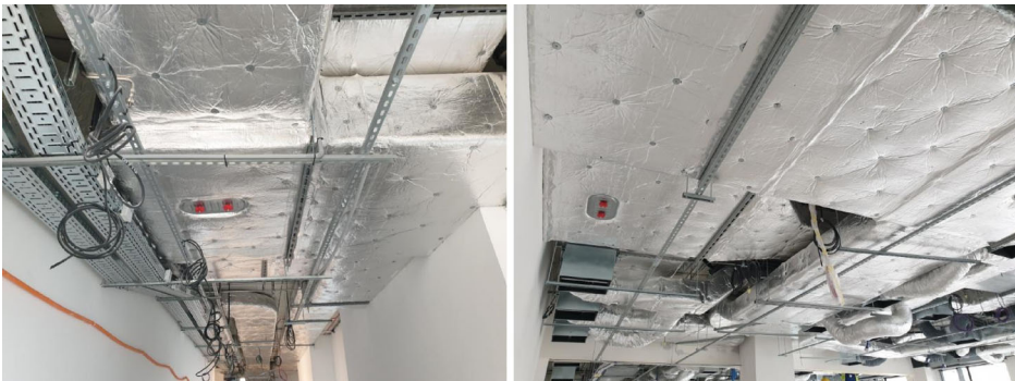
Figure 3. Ductwork underneath a ceiling of a corridor (left) and office space (right). A large amount of ducts reduces the available space for the smoke reservoir. Due to physical limitations, the space available for ducts may be a limiting factor for the design of a smoke control system (Courtesy of R. Brzozowski).
