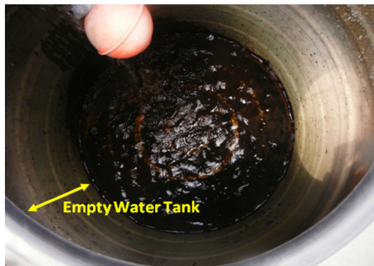
Figure 2. Empty overhead water tank for fire fighting (Color figure online).
