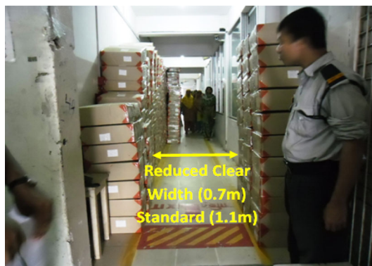
Figure 1. Clear width of an exit corridor reduced by piled up boxes (Color figure online).
