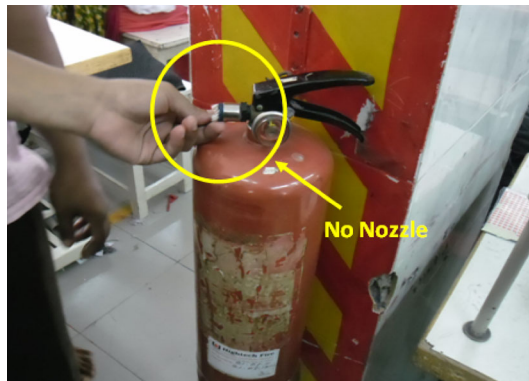
Figure 4. Fire extinguisher with no nozzle (Color figure online).
