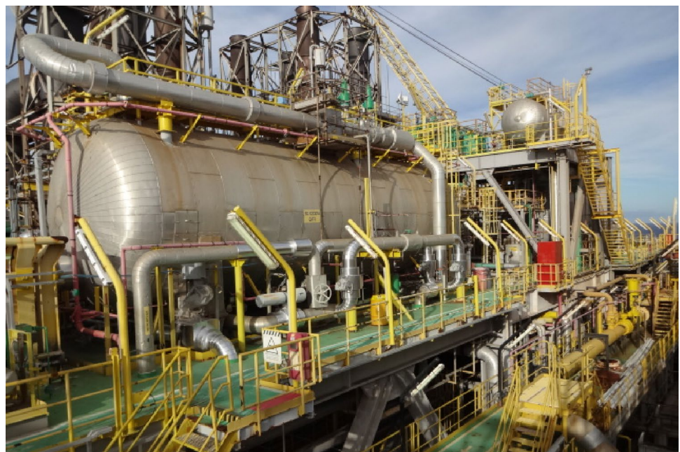
Fig. 1 Process plant of the power generation unit in a FPSO. Source: Authors (2021)
