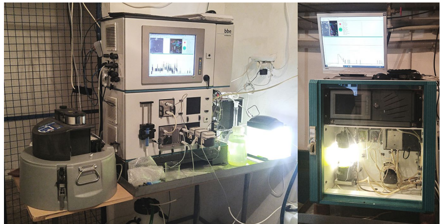
Fig. 3 Monitoring devices installed at the Želivka Water Treatment Plant (left, DaphTox II; right, DaphTox I)
