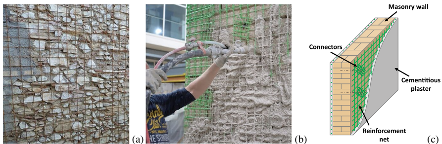
Fig. 1 Application of reinforced plasters to masonry walls: a electro-welded steel net; b GFRP; c scheme of arrangement of the reinforcement
