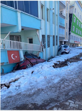
Excessive settlement, bearing capacity failures, soil ejecta at Lat:37.788°N, Long:37.642°E
