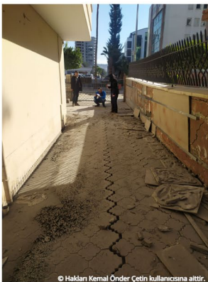
Soil Ejecta, excessive settlement at Lat:36.590223°N, Long:36.177023°E
