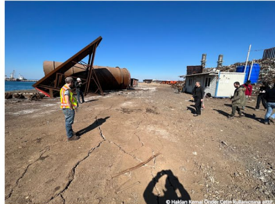
Lateral spreading at Lat:36.778661°N, Long:36.202563°E
