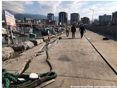
Lateral spreading, excessive settlement at Lat:36.593308°N, Long:36.175766°E
